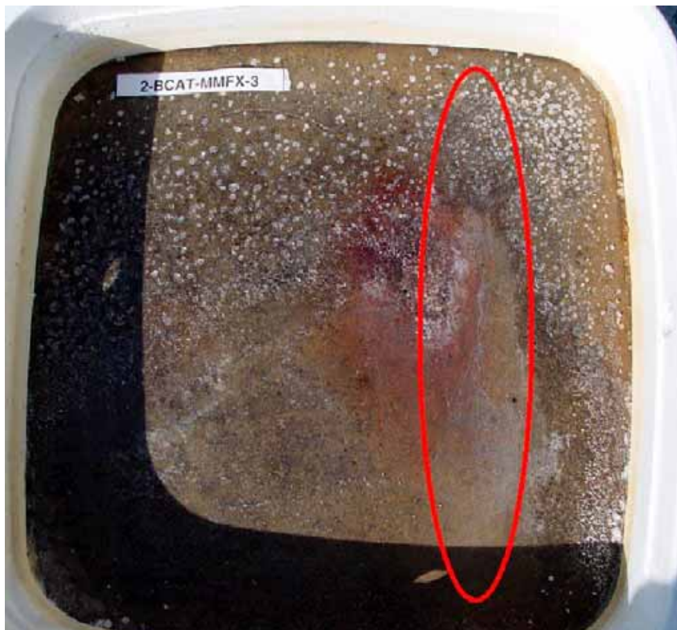
Figure 4.57. Photo. Top surface of specimen 2-BCAT-MMFX-3 after 461 days of exposure.
