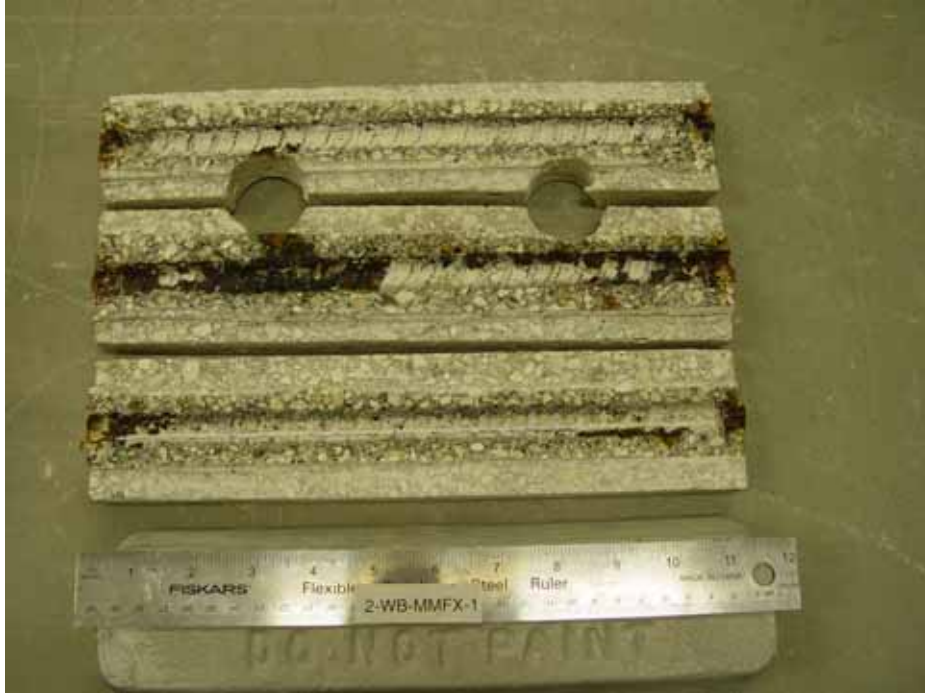
Figure 4.60. Photo. Trace of the upper rebar and corrosion products on specimen number 2-WB-MMFX-1.
