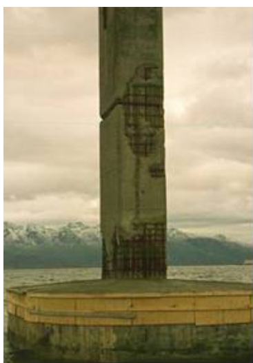
Figure 1-1: Corrosion damage on bridge pier.
