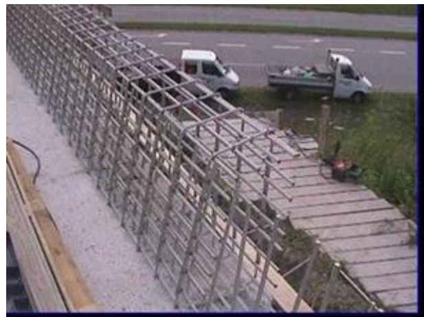
Figure 7-6: Replacing edge beams and parapets on bridges in Denmark exposed to de-icing salt.
