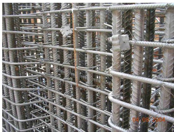
Figure 4-4: Bridge column in marine environment reinforced with two or more layers of reinforcement. The outer layer is SSR and the subsequent layers are ordinary carbon steel reinforcement.
