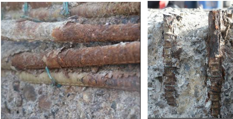
Figure 6-2: Illustration of the adverse corrosion protection performance of epoxy coated reinforcement in the vicinity of the saline waters of the Arabic or Persian Gulf under hot and humid environments.
