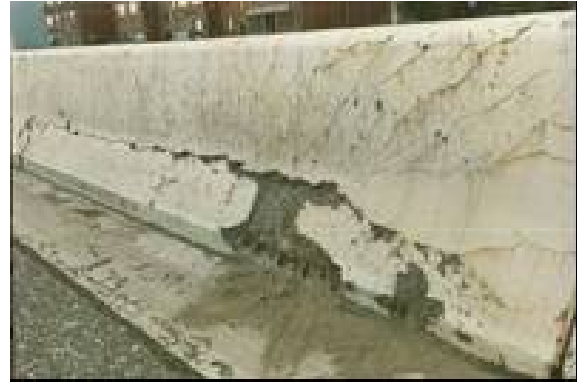
Figure 1-4: Corrosion damage on New Jersey type crash barrier
