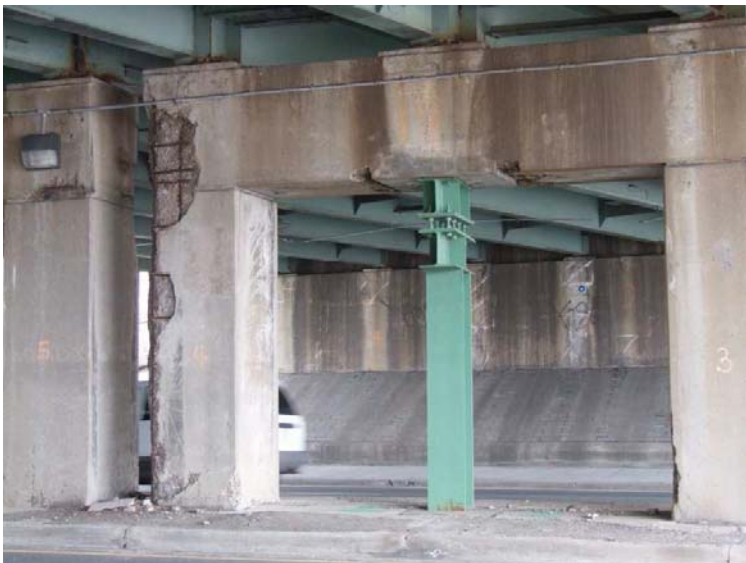
FIGURE 1 Spalling of the concrete as a result of traditional steel reinforcement undergoing corrosion after years of exposure to salt.
